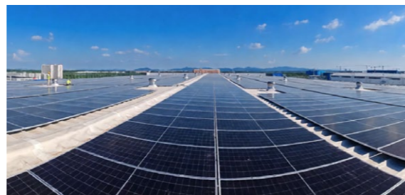
Distributed Photovoltaic System at Nanjing Jiangning Park
