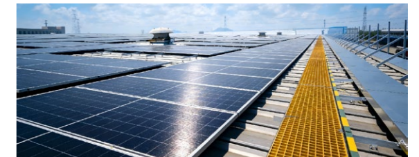
Distributed Photovoltaic System at Wuxi Huishan Park
