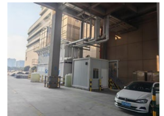
Centralized Refrigeration Unit
