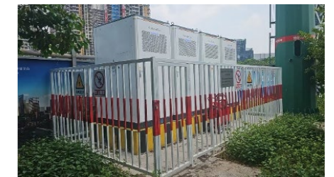
Energy Storage Power Station
